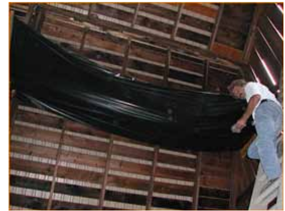
MODIFICATIONS FOR BAT ROOST SITES: TARP HUNG TO PREVENT GUANO FROM FALLING ON HAY. PHOTO CREDIT JULIET CRAIG.
