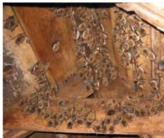
BAT COLONY IN AN ATTIC. A ONE-WAY EXIT DEVICE INSTALLED AT THE CORRECT TIME OF YEAR MAY BE AN APPROPRIATE APPROACH TO EXCLUDING BATS. PHOTO BY JULIET CRAIG.
