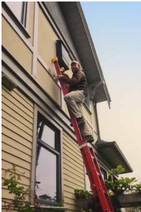
A BIOLOGIST INSTALLS A BAT HOUSE ON THE SIDE OF THE BUILDING PRIOR TO SEALING THE ROOST. PHOTO BY KATIE BELL.
